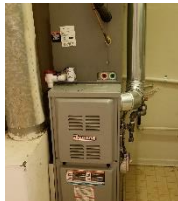
NEW Furnace and A/C
