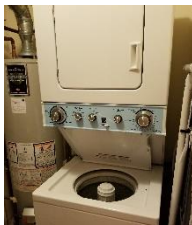
NEW 2017 Hot Water Heater and Washer and Dryer
