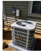
New Air Conditioner
